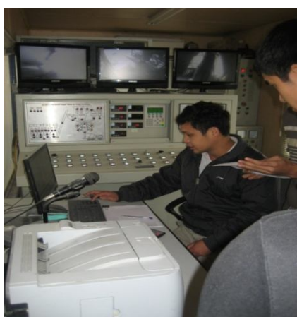
Figure 2 Remote Control Room
