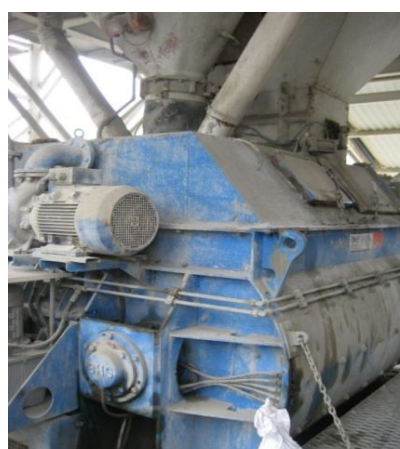
Figure 3 Mixer 4500/3000BHS, Capacity 180 m 3 /hr.
